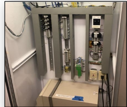
SCADA Control Panel
