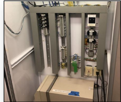
SCADA Control Panel
