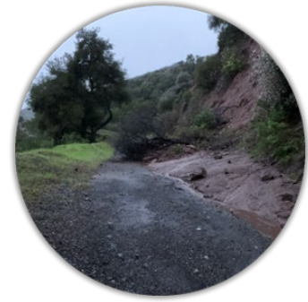
Figure - Glen Annie Road Damage following January 2023 Winter Storms
