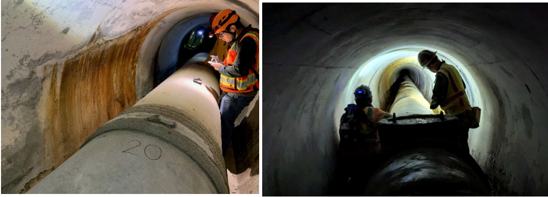
Figure 2. Tunnel entrants inspecting Sheffield Tunnel at Pipe Section #20 (left) and looking west through the tunnel at the first manhole from the east portal (right)
