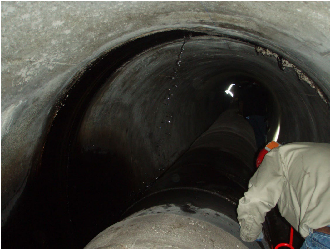
Figure 3. Sheffield Tunnel Seepage
