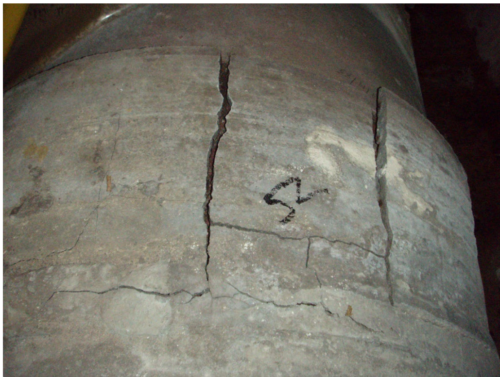
Figure 2. Centrifugal Concrete Pipe Joint Within Sheffield Tunnel Showing Major Cracking
