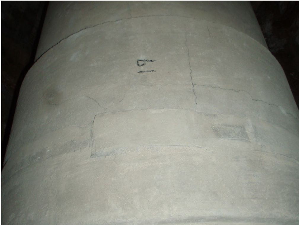
Figure 1. Centrifugal Concrete Pipe Joint Within Sheffield Tunnel Showing Minor Cracking
