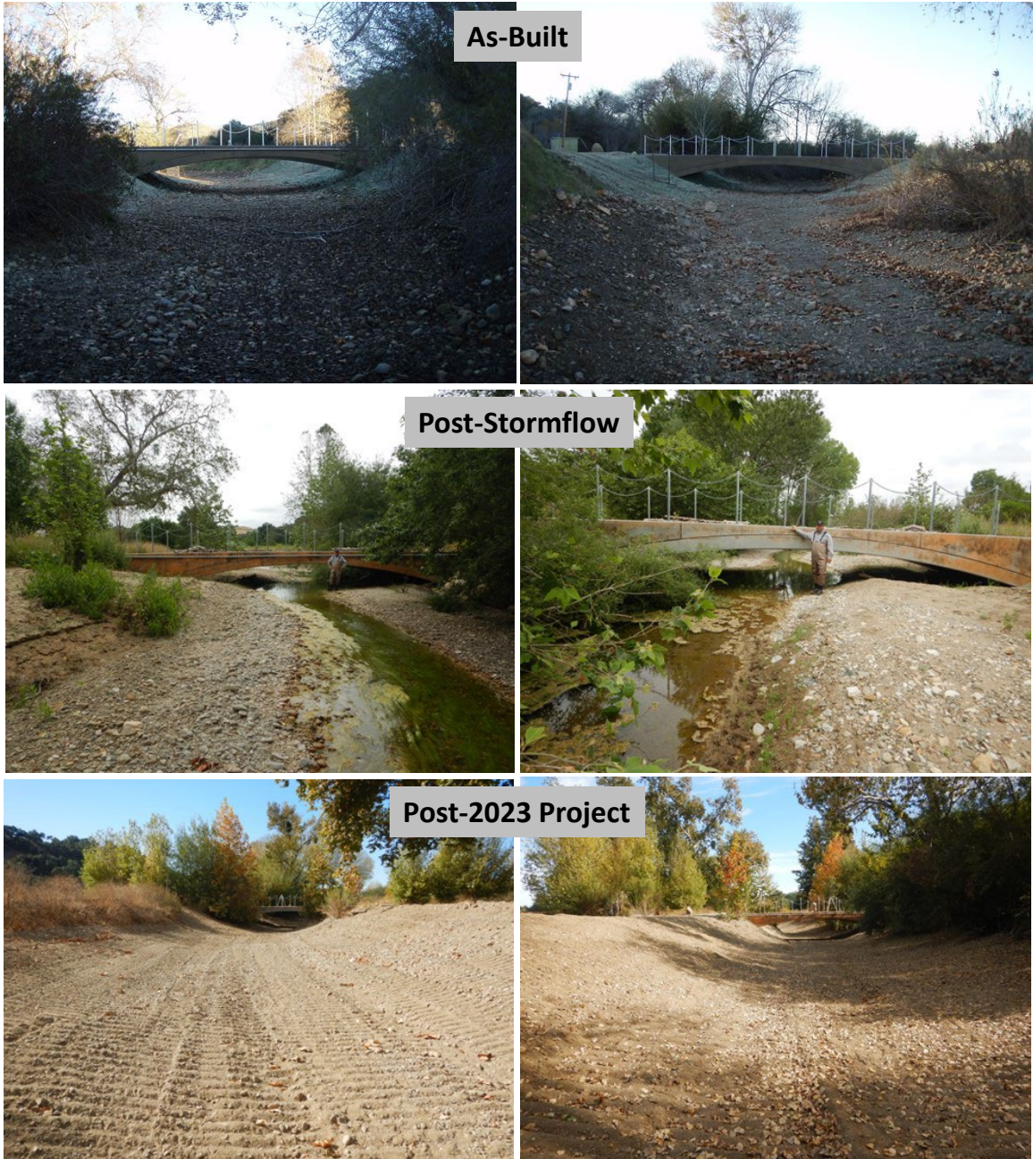
Figure 128: Quiota Creek Crossing 0A showing the As-Built, post-stormflows and post 2023 project conditions.
