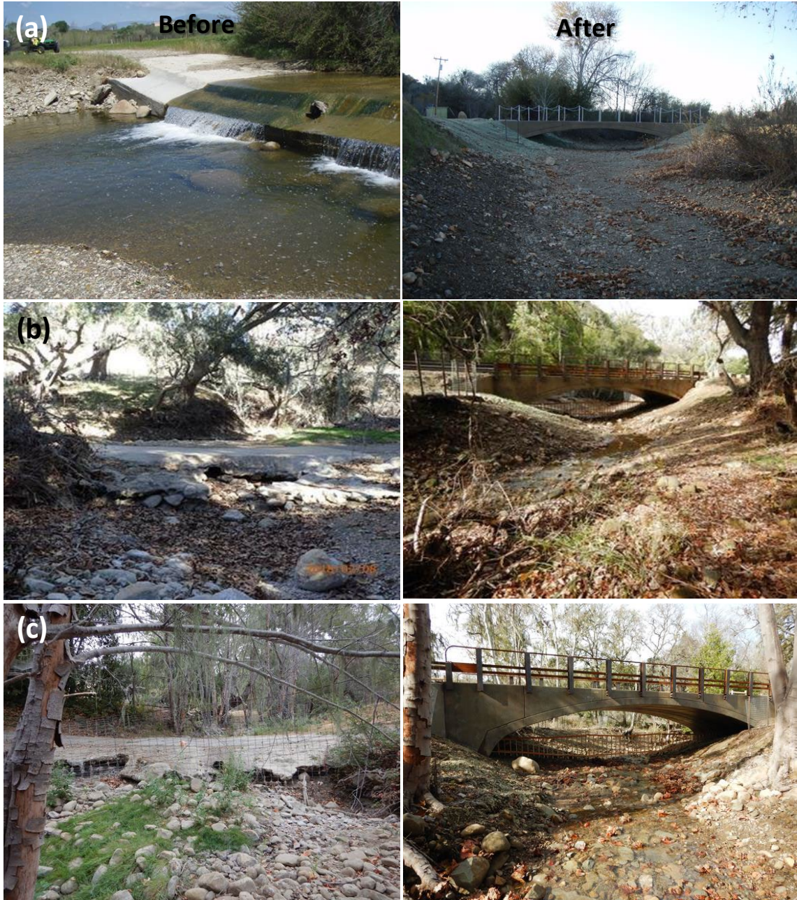
Figure 122: Fish passage and habitat restoration at (a) Quiota Creek Crossing 0A (2015), (b) Quiota Creek Crossing 5 (2018), and (c) Quiota Creek Crossing 9 (2018).
