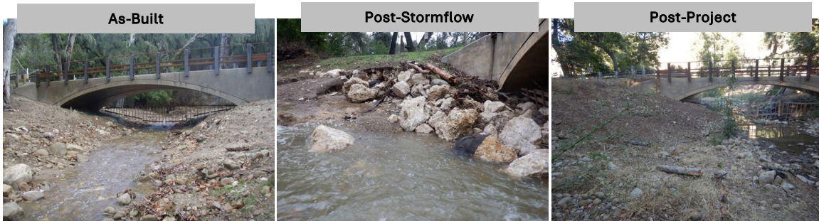
Figure 130: Quiota Creek Project at Crossings 4 showing the As-Built, post-stormflows, and post 2024 project.
