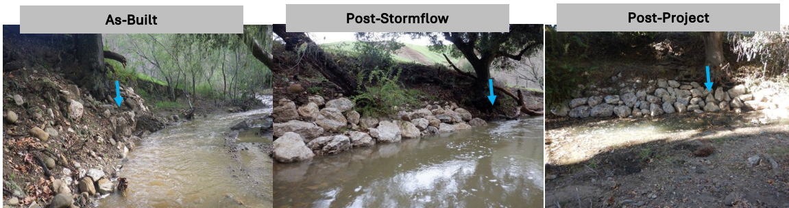
Figure 131: Quiota Creek Project at Crossing 3 showing the As-Built, post-stormflows, and post 2024 project.
